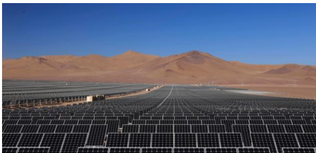
Photovoltaic park in the Antofagasta region (@Acera AG)
