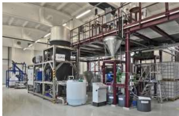
Fig. 1: K-UTEC's technical centre, with more than 1,500 sqm for process technology equipment and systems that can be flexibly combined to replicate complete production processes. The industrial scale demonstration plant allows to process several tons of raw materials into desired end products.
