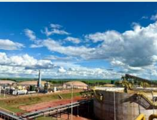
Figure 1 - The image shows Cocal's production site in Paraguaçu Paulista- SP, featuring biogas facilities and CO 2 capture technology.
