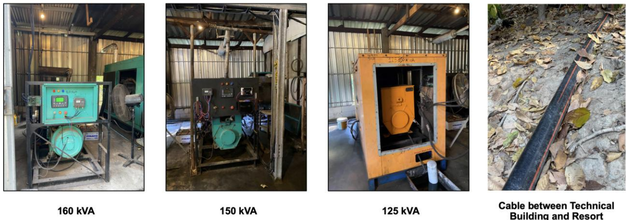
Figure 10. Three diesel gensets and connecting cable between the technical building and the resort (Source: EGS-plan (Bangkok) Co., Ltd.)
